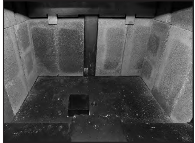
Figure 25: Firebox floor with ash dump.
